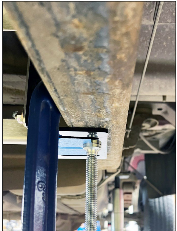
INSIDE / BRACKET EXTENDED AWAY FROM FRAME
