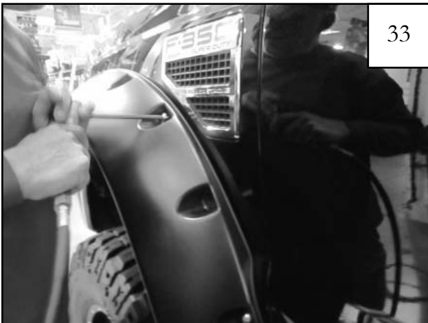
Using torx bit (SW1-0052), start bolts installed in Step 31 through holes drilled in Step 28. Once all bolts are in place, tighten all screws.
