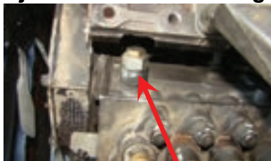
Figure 46 Return Line From the P-7100 Pump
