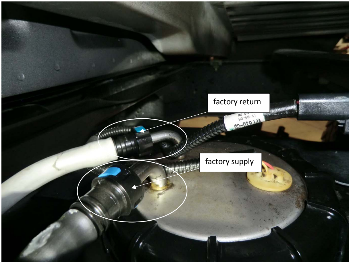
Fuel Supply/return line shown in Photo above.
